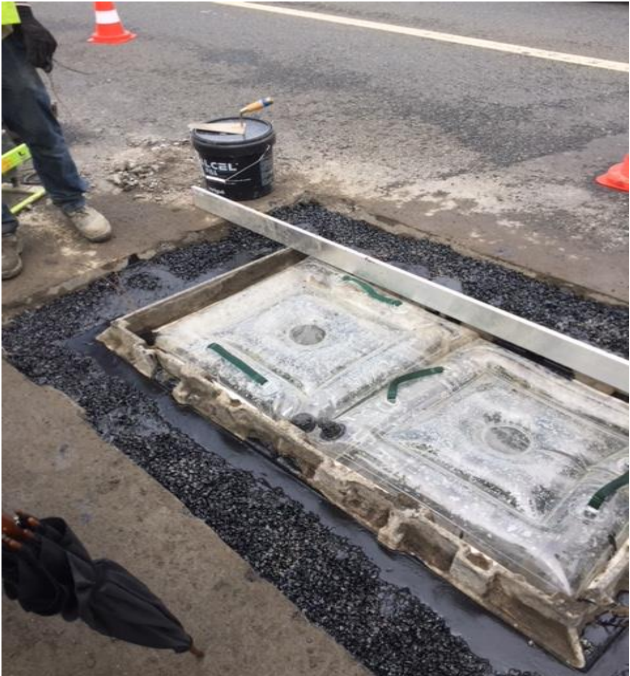
Two pneumatic formwork used to anchor a rectangular manhole on the telecommunication well with the use of polyester resin masses.
