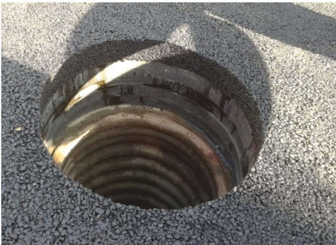
Surface finial of Tegra 600 well made from TVR T System elements (T1/700/50 compensation rings and TXS/700/80 leading ring) prepared for the installation of self-levelling manhole. Jelenia Góra-S-3.
