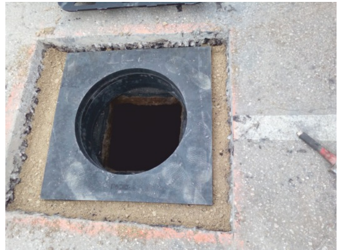
T04/850/620/50 foundation slab installed on T1/600 compensation rings and surface substructure, prepared for assembly of a manhole with 850x850 square plate.
