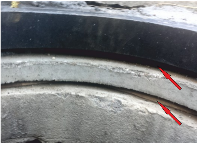
❗ Unacceptable lack of support for compensation rings, adapters. Finial does not provide load-bearing capacity, tightness, and safety of the structure!
