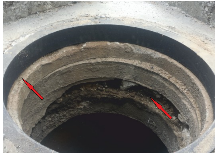
❗ Incorrect ring arrangement (lack of centricity), lack of correct support between the elements
