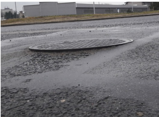
Manhole elevated over the road surface level due to surface's settlement
