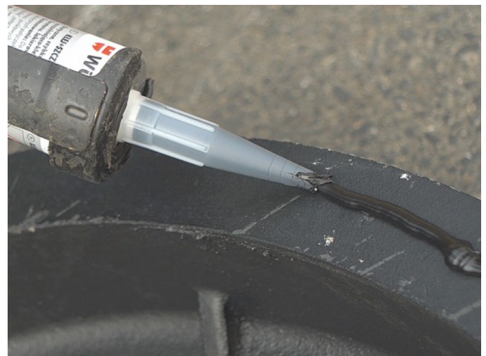
Application of a sealing and binding polymer mass on the surface of lower load-bearing plate of a sewage manhole
