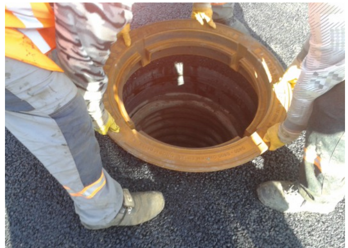
Self-levelling manhole installed in a fortified asphalt surface with the use of TVR T System elements used for construction of Tegra 600 plastic surface well. Jelenia Góra-S-3.
