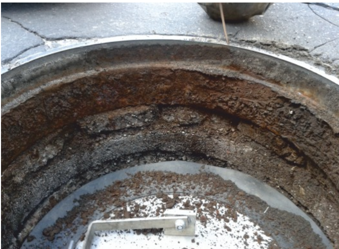
Degradation of a structure supporting a manhole. Concrete mortars in a not bound state and cracked compensation rings. Finial has no tightness and load-bearing capacity.
