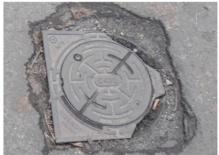
⚠ Telescope manhole for DN315 well damaged due to the lack of even and permanent support.
