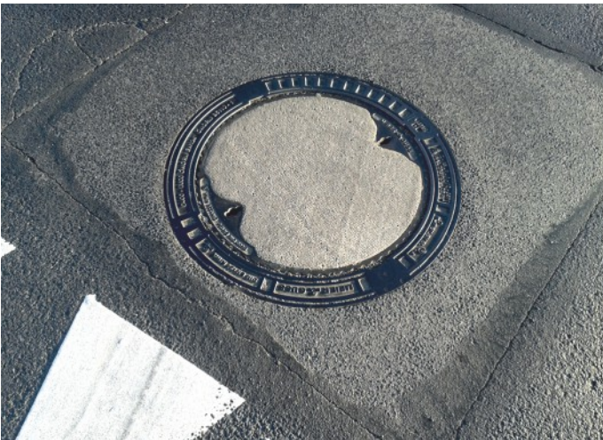
Surface finials made using T1/700 compensation rings and TXS/710/80 adapter that allow to install the self-levelling manhole. Legnica, road S-3, cross ride on manhole, traffic load of Kr 4 lane. 9 years of operation.
