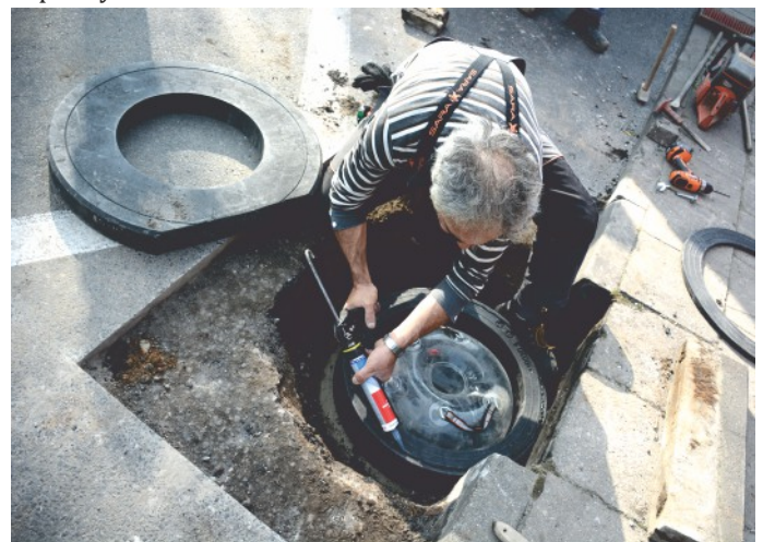
Application of polymer masses between the elements of rehabilitated street drain surface finial.
