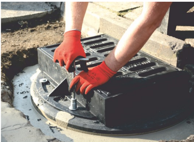
400x600 street drain, flange 3/4, installed on a TX/765/410/80 adapter. Drain anchored to the adapter. Adapter is secured with poured mass poured around the repaired finial. Poured mass constitutes as a substructure for road surface.
