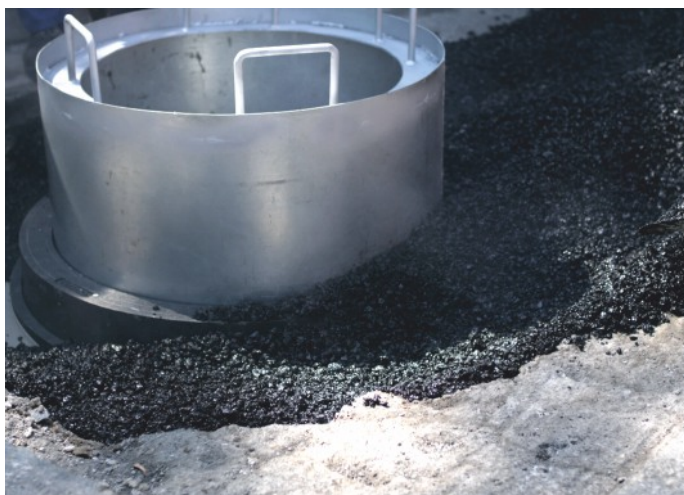
Preparation of a structure supporting self-levelling manhole made from TVR T System elements and hot asphalt mass. The temperature of asphalt mass (170° C) has no influence on the parameters of compensation and leading rings during the installation.
