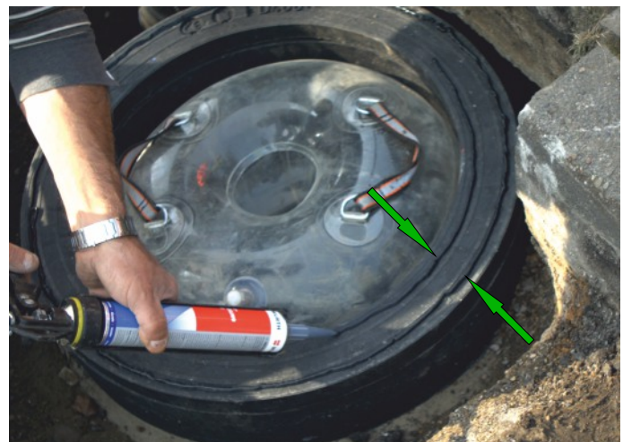
① Application of flexible sealing and binding polymer mass between all the adjustment elements and cast-iron.
