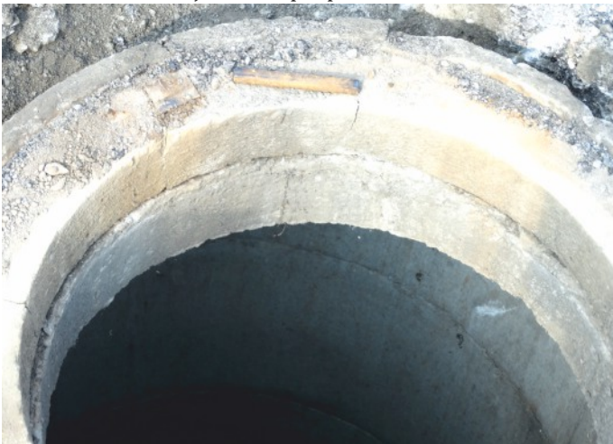
Degradation of structure supporting the manhole. Reinforcement rods as a compensation material - destructive point pressures.
