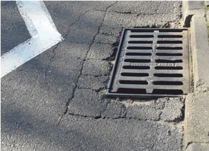
Exploited roadway drain. Location is unfavourable - buses regularly ride over the drain. Surface cracks are caused by the lack of finial tightness and lack of substructure.
