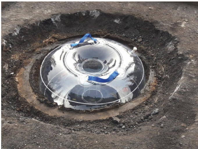
Before commencing the disassembly works of a finial, the pneumatic formwork can be used as a protection against contamination.
