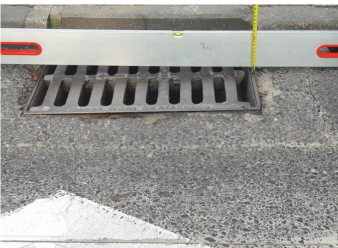
Verification of technical condition of a drain. Drain is collapsed. The grate in the frame is lowered.
