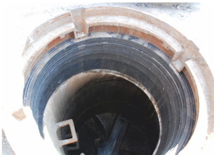
① Structure of a tight surface finial of concrete well with DN625 manhole opening made only on the base of TVR T System plastic rings. Height adjustment of 24,3 cm that refers to surface inclination angle. Lack of joints based on cement mortars. Polymer masses are used as sealing material.
