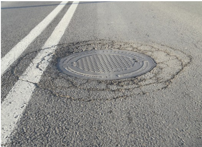
Finial of a sewage well located centrally in the line of vehicle wheel ride. Kr 2-3 traffic load. Elements supporting the manhole are degraded, substructure is damaged, and road surface is cracked.
