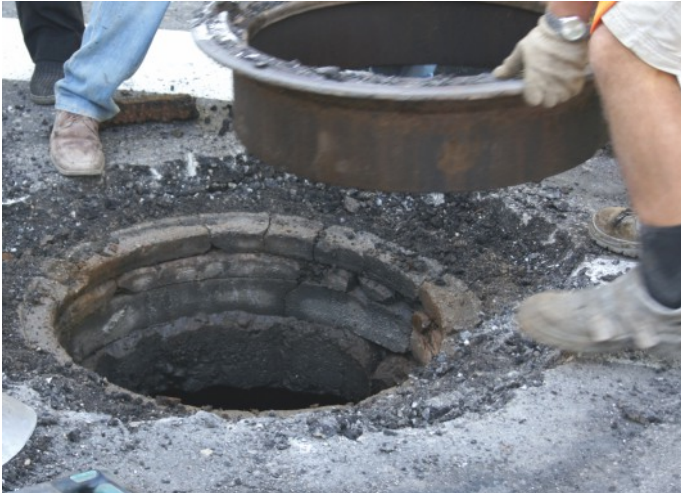
Disassembly of a self-levelling manhole with smaller frame support surface (about 1600cm 2 ) installed directly on concrete elements! Negative weather conditions. Operation period 1.5 year
