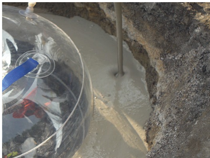
Pu-TS 625 formwork installed in a manhole opening of a well allows to pour the compensation layer.
