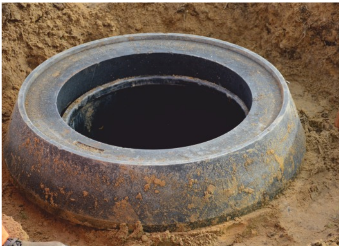
T3/615 relief cone securing a shaft pipe of DN600 well.
